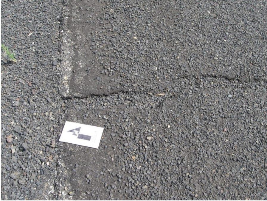
Figure 19: A photo of the surface of W Yakitat Road showing an open tension crack in the asphaltic concrete pavement. The road was recently (prior to my August 2013 visits) paved with chip seal, seen as the black gravel on top of asphaltic concrete pavement and in the tension crack. This particular crack is located on the edge of the northern shoulder of the westbound lane uphill of the buttress. Scale arrow faces north. The black fields on the scale measure 1.96 inches (5 cm). Photo was taken August 2013.
