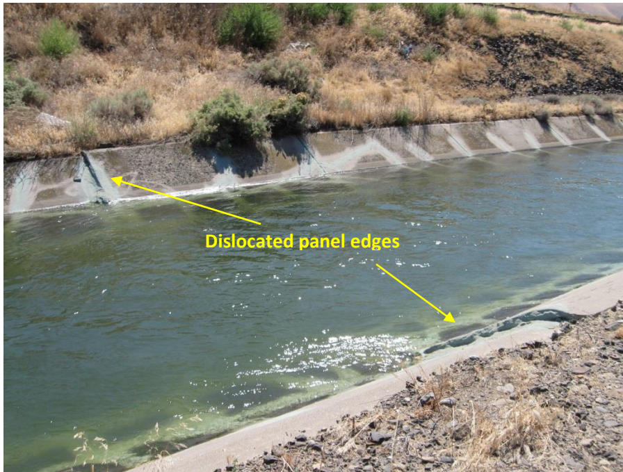
Figure 20: A photo of the KID canal taken during August 2013 showing an unlined section. The panel at the center of the photo has been dislocated from its original position. The KID reported that this was due to frost heave. Canal joints have been sealed with a green substance.
