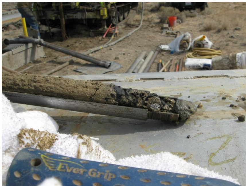
Figure 21: A photo of the silty clay and gravel with matrix contact taken immediately after the split spoon sampler was opened. Sample is D-8 and was taken at a depth of 28 feet from borehole H-101vwp-13.
