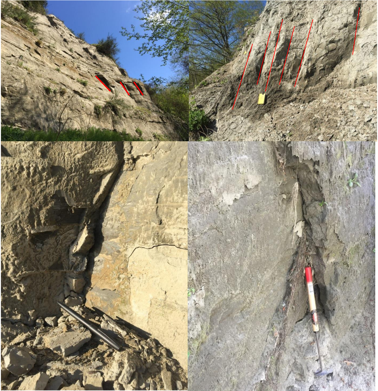
Figure 11a (upper left): inaccessible joints marked out in red at the southeastern end of the study area. Figure 11b (upper right): a joint set marked out in red and oriented parallel to the local bluff face at the northwestern end of the study area.
