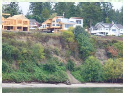
Fig. 3: A recent landslide near on south Whidbey Island, near the Clinton ferry terminal. Quantitative assessment of shoreline retreat is very important for areas, such as this location, where shoreline development is occurring.
