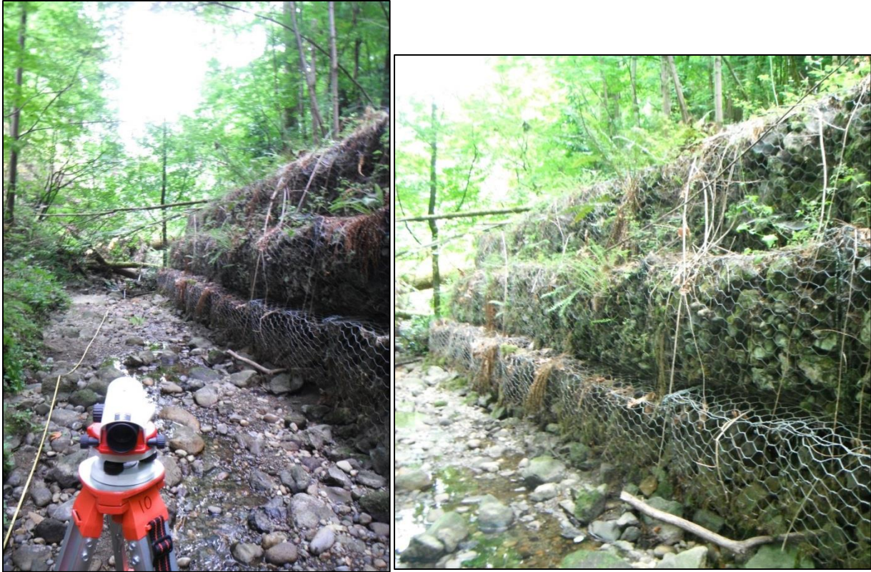
Figure 16. Photo of a gabion wall that was installed to stabilize the west slope. Undercutting by the stream has led to angular blocks falling out from under the wire.
