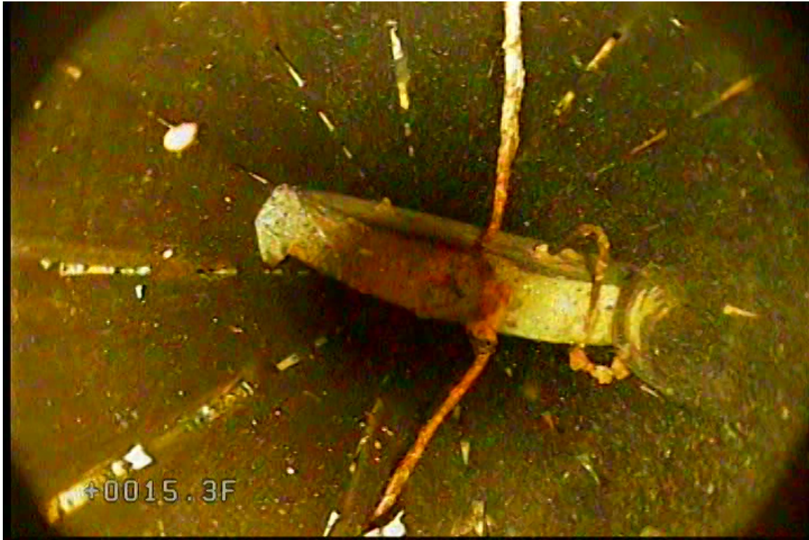
Figure 3-2: Well 6. Obstruction, possibly part of dislodged end plug at ~ 21.7 ft depth.
