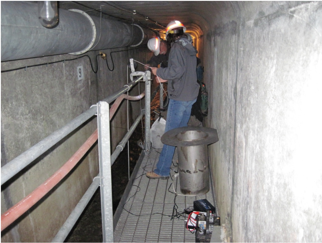
Figure 3-1: USACE Geologists using a downhole camera to record the condition of the relief wells in the 6-ft high section of the tunnel.
