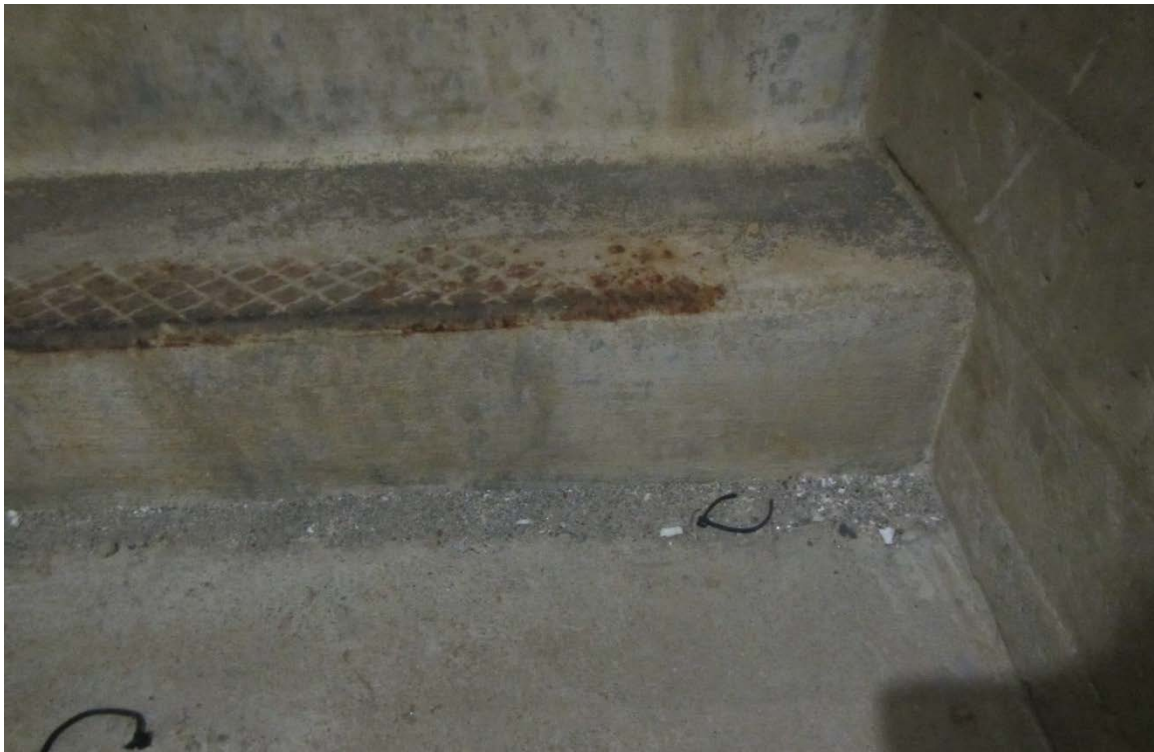
Figure 3-5: Sediment accumulating below stairs.
